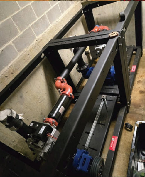
ABOVE The Richard Meier building elevator, which transports visitors and large works of art, now has an updated electrical and mechanical system.
